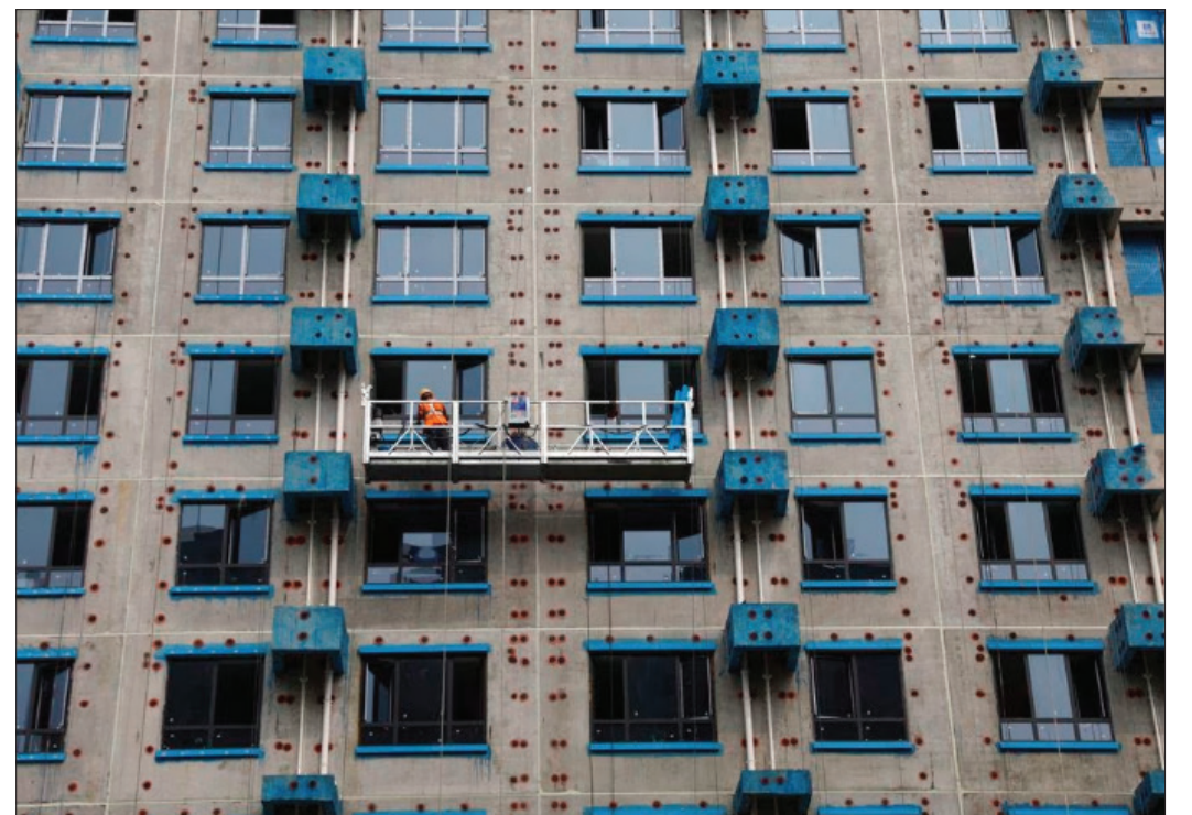
A person works at a residential building construction site in Beijing, China. The world's second-largest economy has been struggling after a brief post-COVID recovery.
